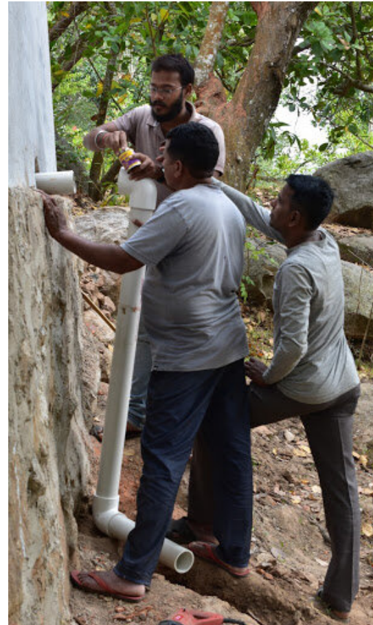
Installation team members connecting the Hydrodoser system to the existing water distribution network.
