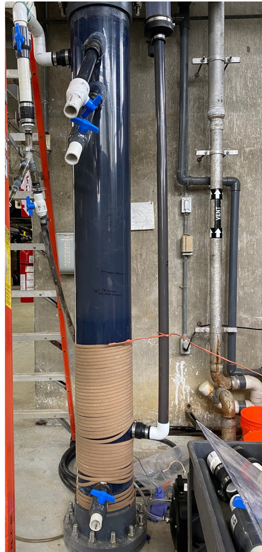
The UASB reactor is wrapped with heat tape to control its temperature at the Ithaca Area Wastewater Treatment Facility (IAWWTF).
